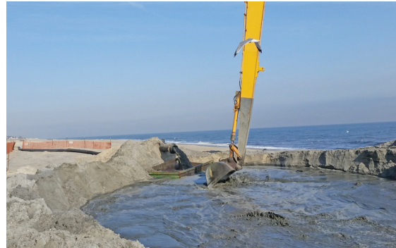
The dredged slurry of 90% sand is pumped through pipelines and is temporarily held in a sludge dewatering zone on the beach so that it can dry and be suitable for placement as beach fill.
